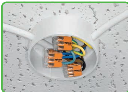
Lighting distribution in ceiling canopy
